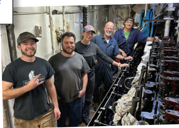
On the Matson vessel RJ PFEIFFER in Alameda, CA, M.E.B.A. Oakland dayworkers assist Wartsila and the vessel's Chief Engineer with camshaft replacement of all three of the ship's diesel generators. Dayworkers left to right are Matt Perry, Alex Dunn, Sabrina Brown and Christian Yuhas. At far right is C/E Pat Preston. The photo was taken by Matson RJ PFEIFFER Port Engineer Kenneth Boothby.
