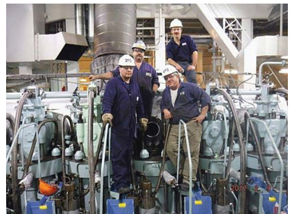
M.E.B.A. engineers changing out the #4 Cylinder Exhaust Valve onboard the OSG tanker OVERSEAS LONG BEACH. Left to right are 2nd A/E Chris Paul, C/E Marc Supersano (top left), 3rd A/E Chris Bolinger (top right) and 1st A/E Chance Parent (front right).
