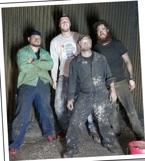
Inside the V2M8 boiler on the MATSON NAVIGATOR following a 20-hour casing leak repair underway. Pictured left to right are 1st A/E Mike Marino, Cadet Damian Dyrdas, 3rd A/E Asher Liss, and EU Jackson Blaty.
