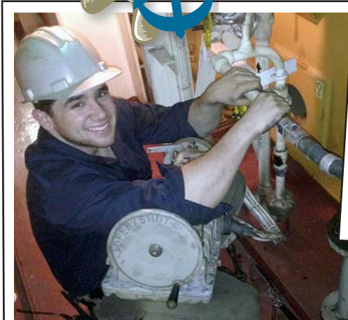
Ben Baitcher, 3rd A/E aboard the USNS WATKINS (Patriot), making repairs to one of the ship's diesel generator cooling water valves.
