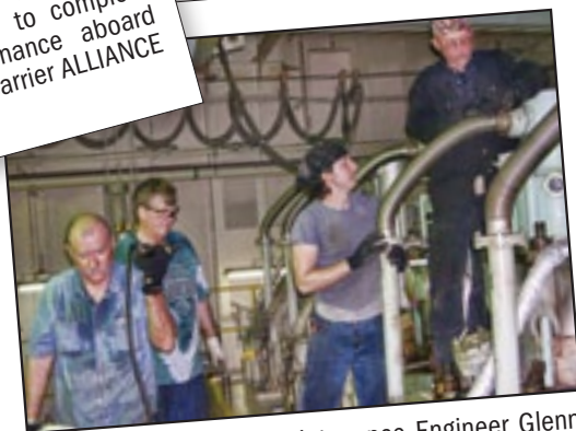
1st A/E John Booth, Maintenance Engineer Glenn Sharp, Cadet Nate Putnam and Maintenance Engineer Matt Miller in Beaumont, Texas preparing to pull a piston head onboard Central Gulf's M/V GREEN LAKE.
