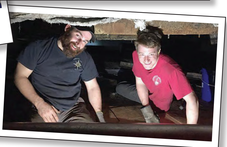
Onboard the HORIZON SPIRIT (Pasha/Sunrise), 2nd A/E Dan Antonellis and Day 3rd A/E James D'Amico were spotted under the boiler repairing a superheater tube.
