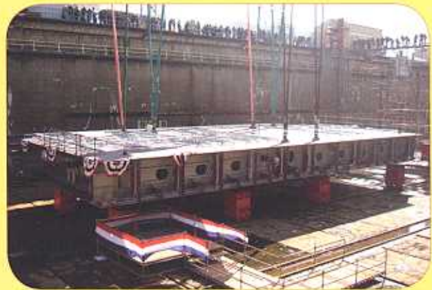
Philadelphia's Aker Kvaerner staged a keel laying ceremony for the first of the double hull product tankers it is constructing for OSG. MEBA's Atlantic Coast V.P. Don Keefe recently locked up a new 10-year contract with OSG covering the existing fleet, MSP ships and newbuilds.
