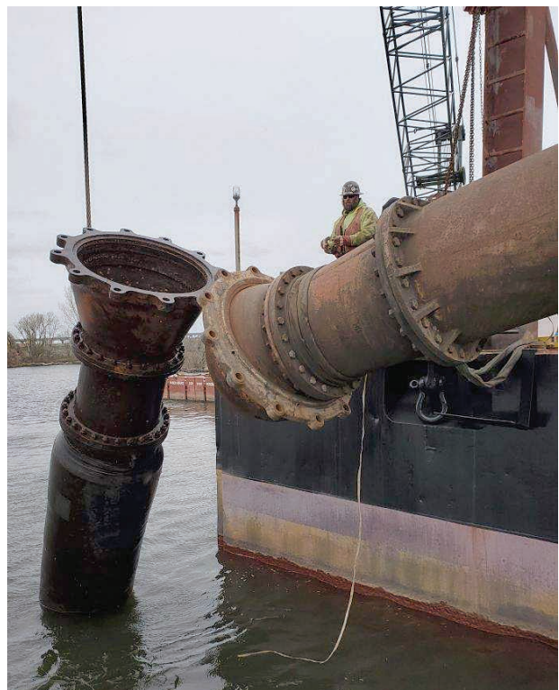
Members working under our contract with Philadelphia Ship Services recently reattached a 48" hose coupler for dredge spoils onboard a U.S. Army Corps of Engineers barge. Members working on that project included Kevin Barry, Chris Grupp, Brendan Joyce and Ryan Grupp.
