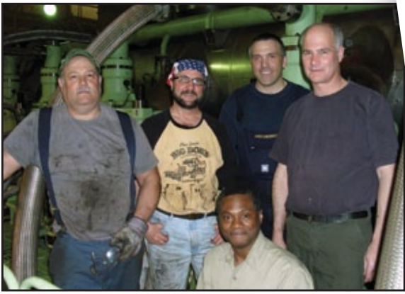
When MLL vessels call in Port Elizabeth NJ, they often request that a team of M.E.B.A. engineers perform needed ship maintenance. The MAERSK IOWA recently passed through and engaged a team of M.E.B.A.'s finest in order to change out a main engine fuel oil pump. Pictured from left to right (standing) are M.E.B.A. Day Engineers Ed Wiessmeyer and Don Raffaniello, C/E Mike Pride and 1st A/E Russ Johansen. Kneeling is Night Engineer Richard Adams.
